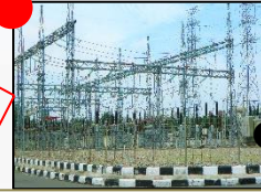
Electricity 150 KV / 60 MVA
