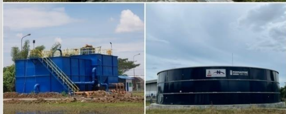
Industrial Water Facilities (WTP) Provider : PT DCC Capacity 500.000 M3/Month
